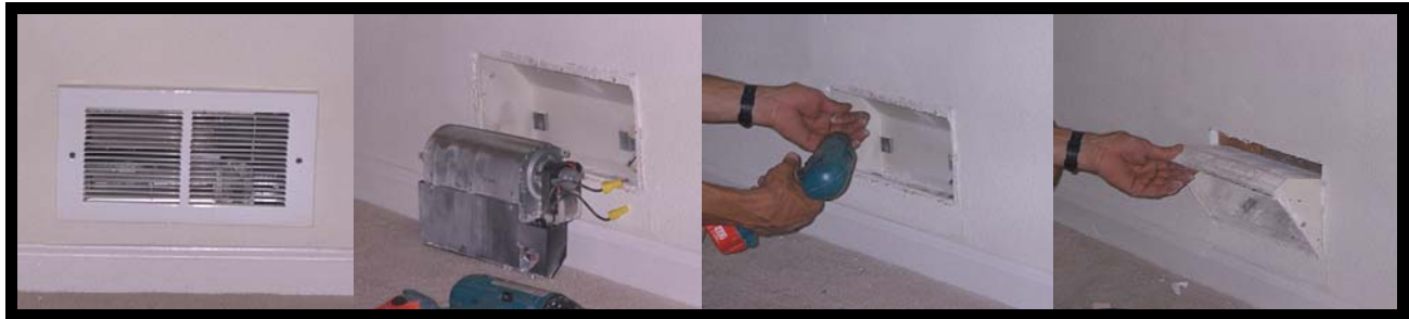
The old heater needing to be replaced.
